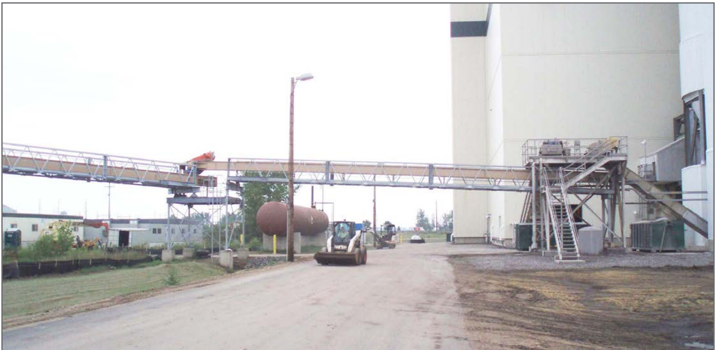
First in the series of En-Masse Drag Chain ash handling system. The structural supports and access towers provide safe and easy access to the conveyors.
